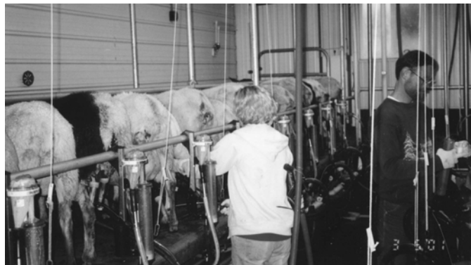
Picture 2. Meter jars installed in a low line pipeline on testing day
